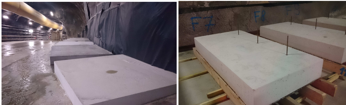
Figure 4. Slabs in place after formwork removal and sidewall with rods used to seal the block in the siding of the access tunnel
